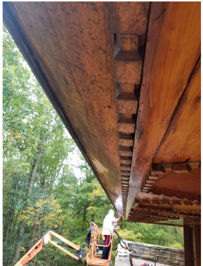
Fig. 11 Image of Finish Failure and Soiled Cypress Fascia Board Source: Image by Author
