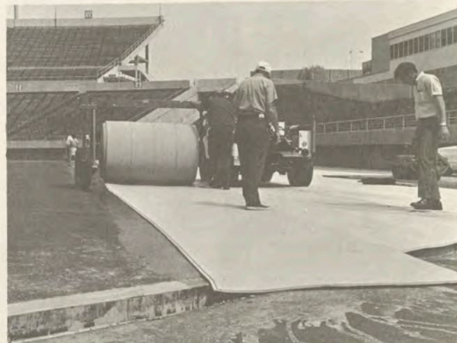
The Monsanto workmen lay the foam rubber padding atop the asphalt surface. The next step is the laying of the turf.
