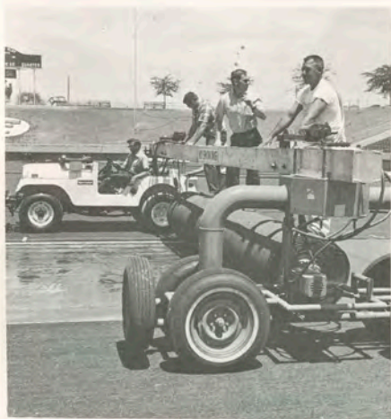
Nearing the last phase of the installation, workmen lay long strips of AstroTurf to cover the field. Next is the stitching.
