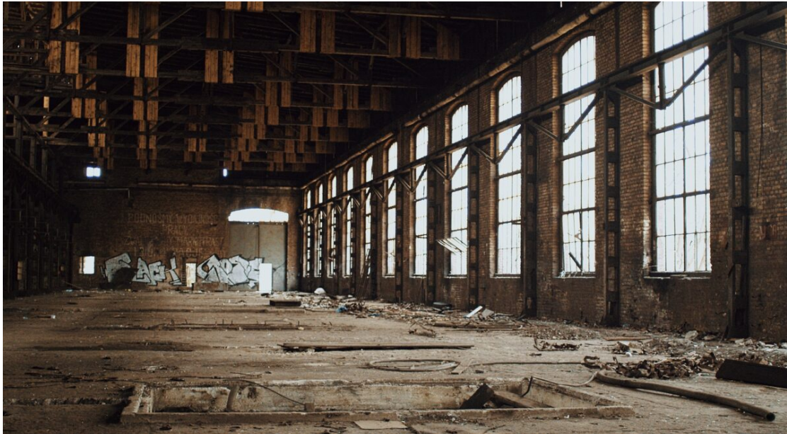
Figure 4 Franczak, Michal. "How to save your city's abandoned factory." Hub, 4 July 2022, https://hubin-project.eu/how-to-save-your-citys-abandoned-factory/ Act two inspiration.
