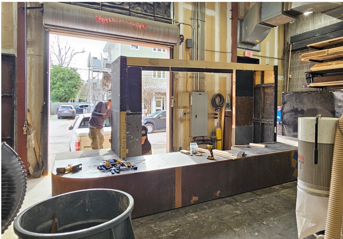
Figure 35: Louks, Kaeanne. Image of the outer deck post-facing and installation of house's base structure from stock platforms in the scene shop. 2024, Tulane University.
