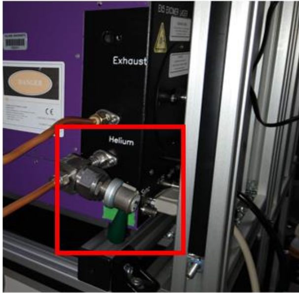
Figure 3-10 External manual valve installed
