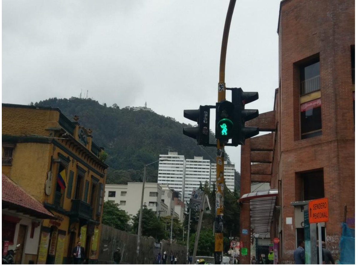
Figure 30: New traffic signal installed along La Carrera Séptima (my own photo)
