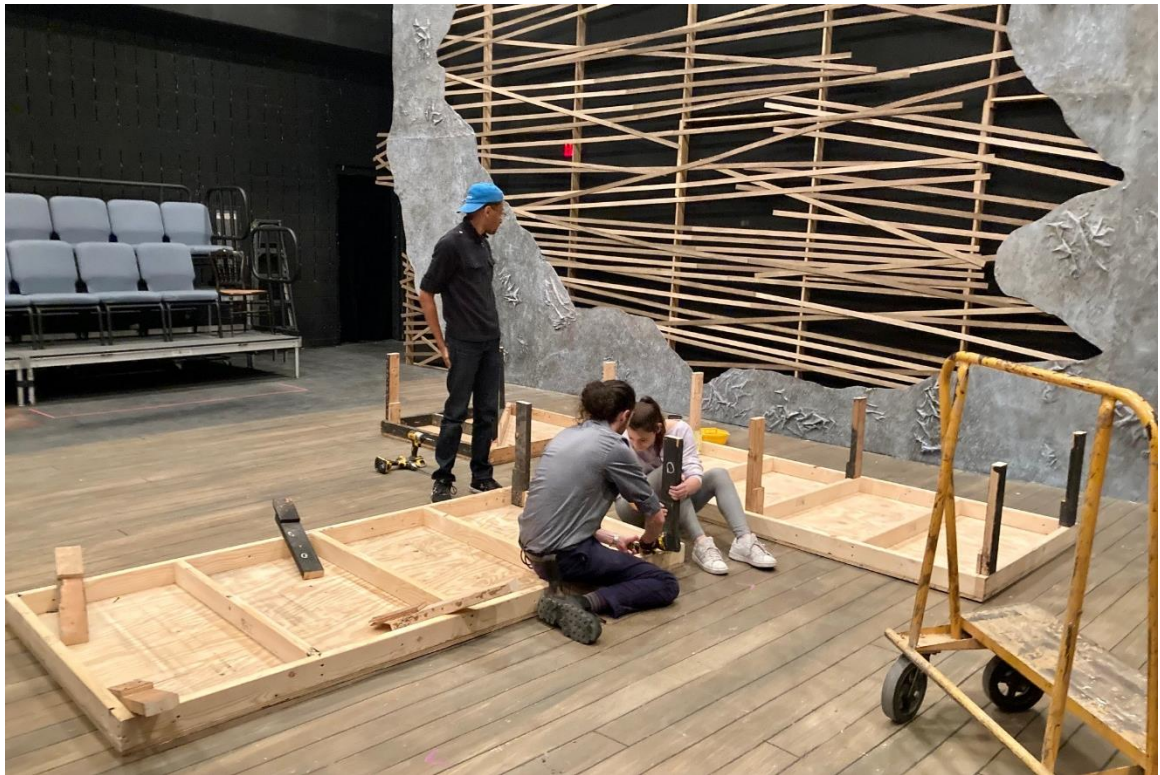
Figure 88: Compression legs are fastened to stock platforms after the voile is installed. 2021, Tulane University.
