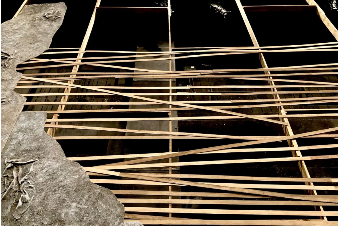
Figure 72: The wooden slats are stapled into place behind the plaster. 2021, Tulane University.
